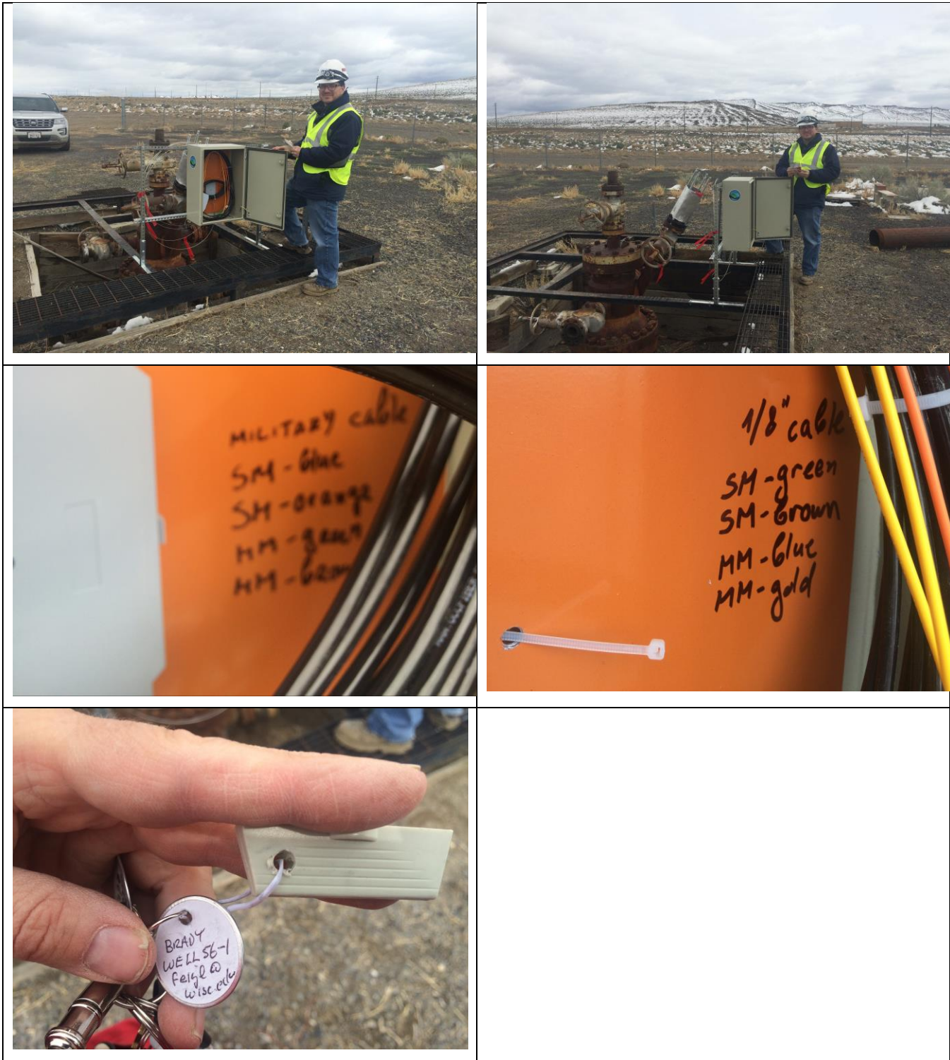
Figure 2. Junction box for vertical fiber optic cable near Brady Well 56-1.
