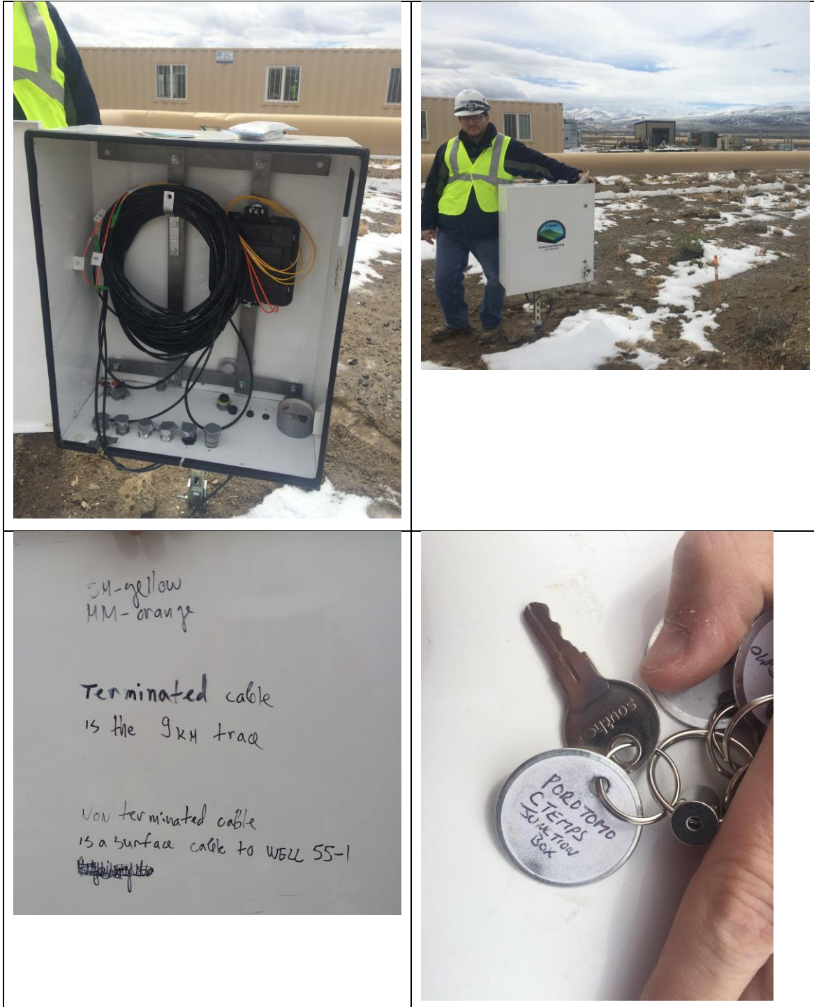
Figure 1. Junction box for horizontal fiber optic cable at Brady Hot Springs, Nevada. Photos taken March, 2016. The temporary container building with windows has since been removed.
