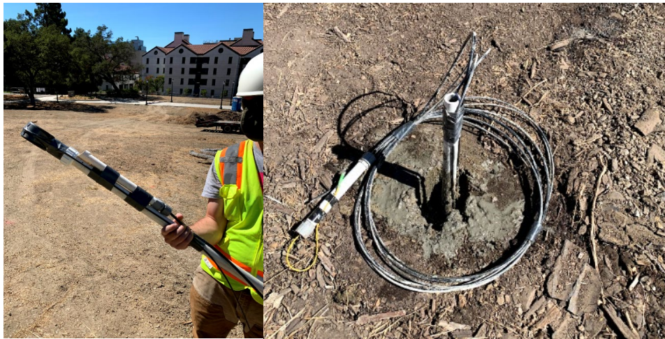
(a) Distributed fiber optic sensor installation
