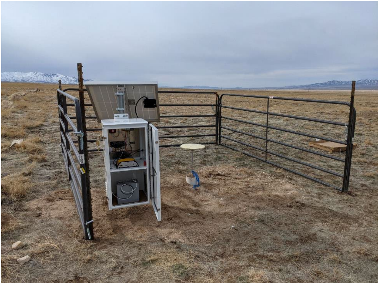
Figure 12: Continuous GPS station, GDM-C1. Installation is west of pad 58-32 embankment.
