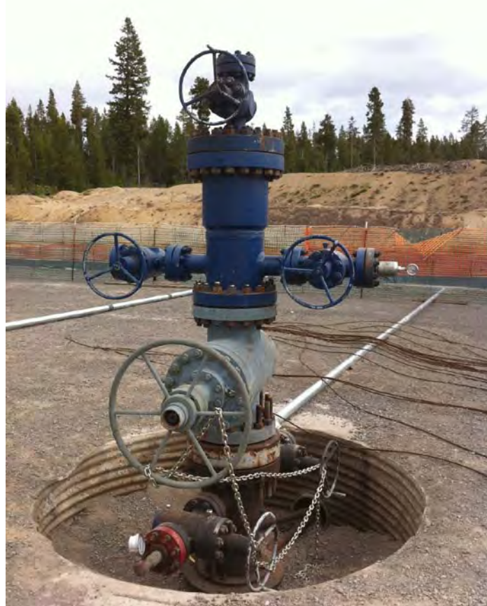
Figure 7-19. Existing wellhead on NWG 55-29. Everything above and including the gray, 12 in master valve will be replaced with a high-pressure wellhead suitable for stimulation.
