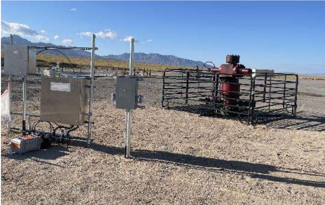
Figure 24. Final installation with Silixa/Baker Hughes enclosures on the Unistrut frame.
