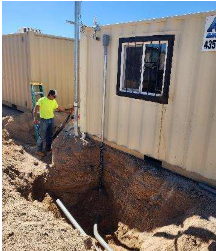
Figure 17. Conduit routing for fiber optic cable into Silixa acquisition trailer.
