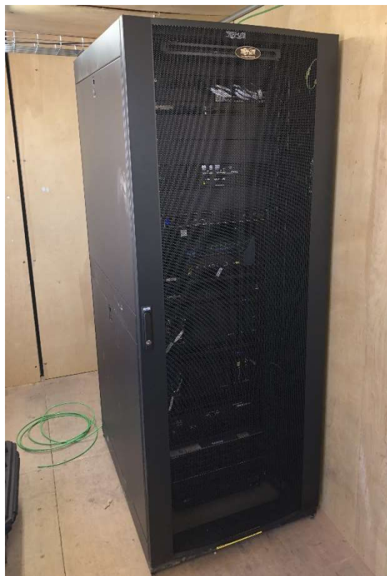
Figure 27. Edge monitoring system cabinet.
