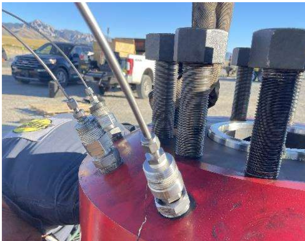
Figure 21. Cables exiting Wellhead Outlets after the wellhead adapter was replaced.
