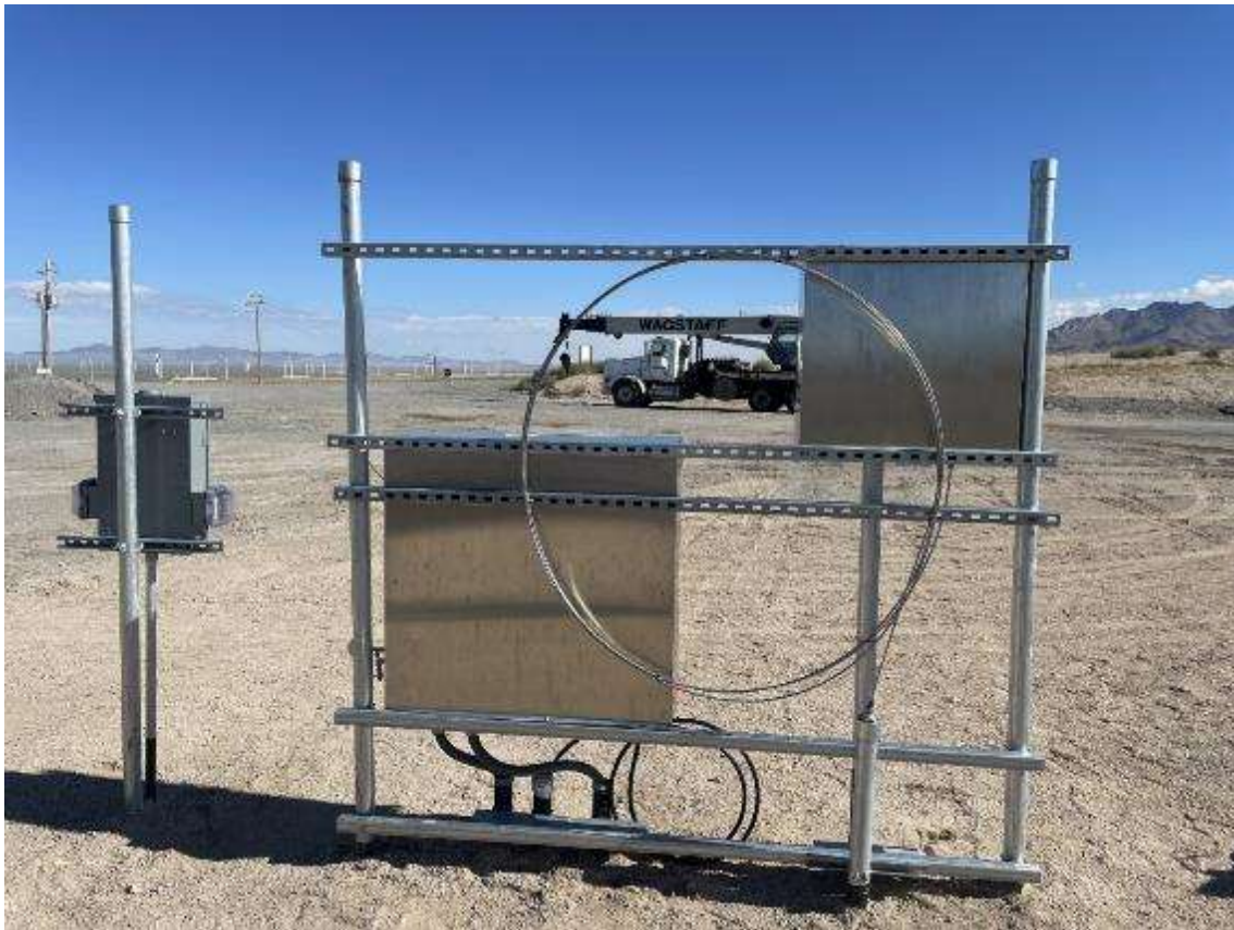
Figure 25. Excess Silixa fiber optic service loops stored on the back of the frame.
